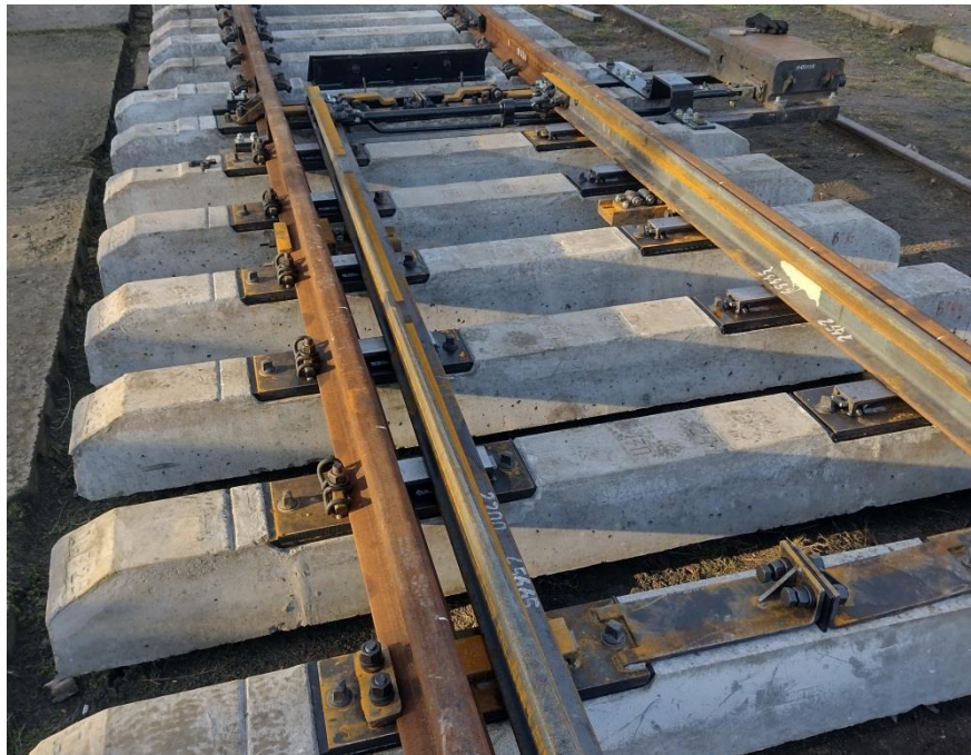
Figure 1. Switch points of a R65 turnout with a 1/11 crossing, track gauge 1 435 mm (Ukraine)
