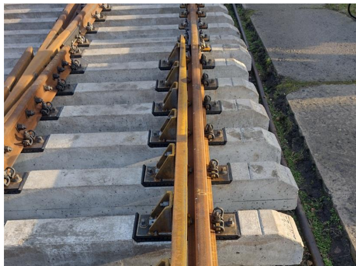
Figure 2. Frog with guard rail of a R65 switch, 1/11 crossing, track gauge 1 435 mm (Ukraine)
