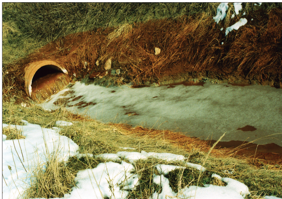
Photo 2. Foamy alkaline water flowing out of leakage of sludge reservoir (Photo by JUHÁSZ, Á. 2003)
