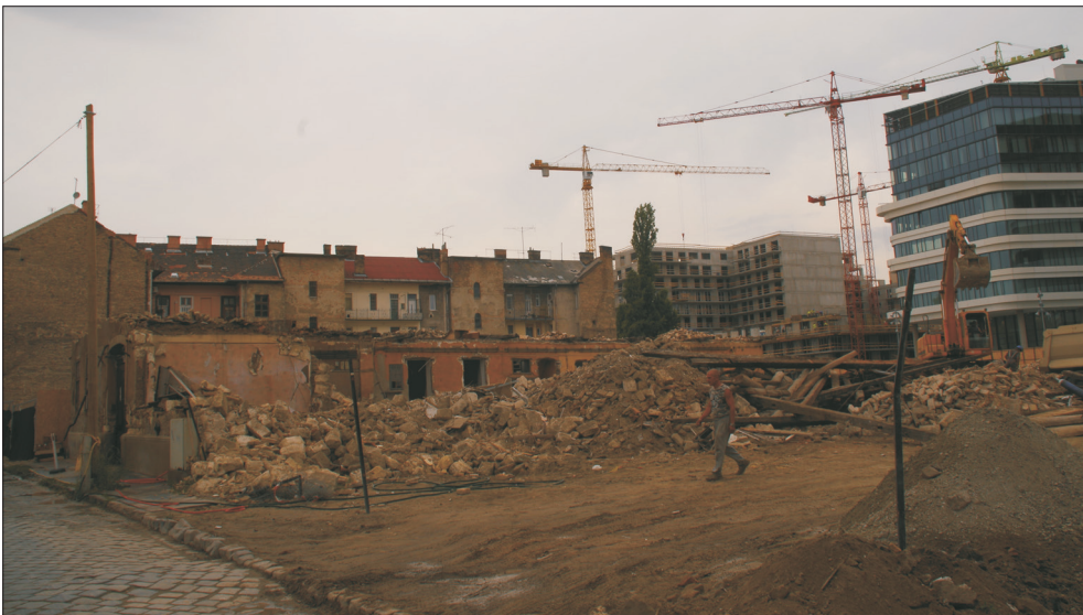
Photo 1. Large-scale, local government initiated regeneration activities in the centre of Józsefváros (Photo by BOROS, L.)
