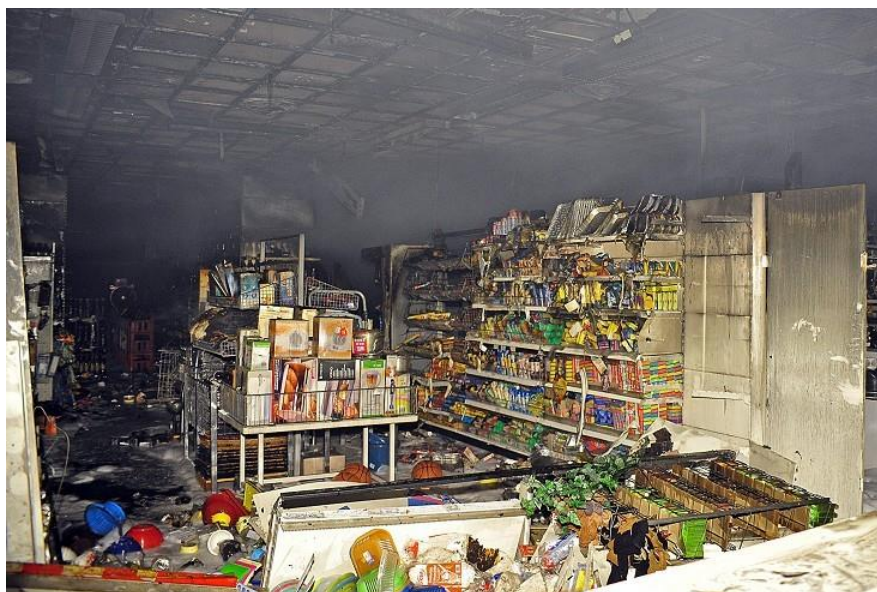
Figure 1: Grocery store sales area after a fire
