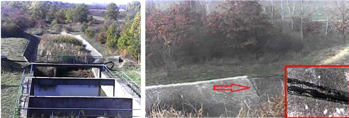
Figure 4 - Photo of the normal floodway of the dam (left) and one of the crack author noticed during the flight (right).
